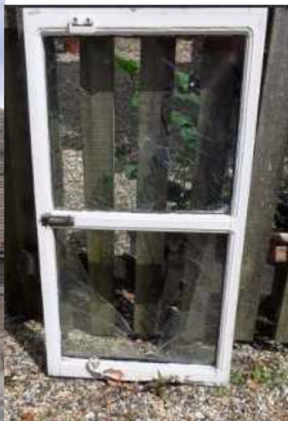
Image, Damage sustained Source: Local trades person
