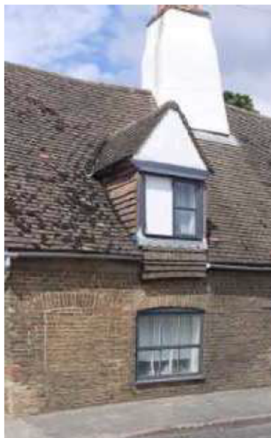
Image, Damaged sustained Source: Local trades person
